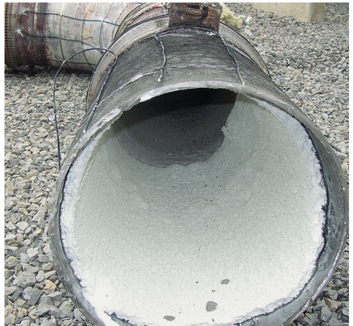
Figure 32: Ammonia salt deposits in a pipe
