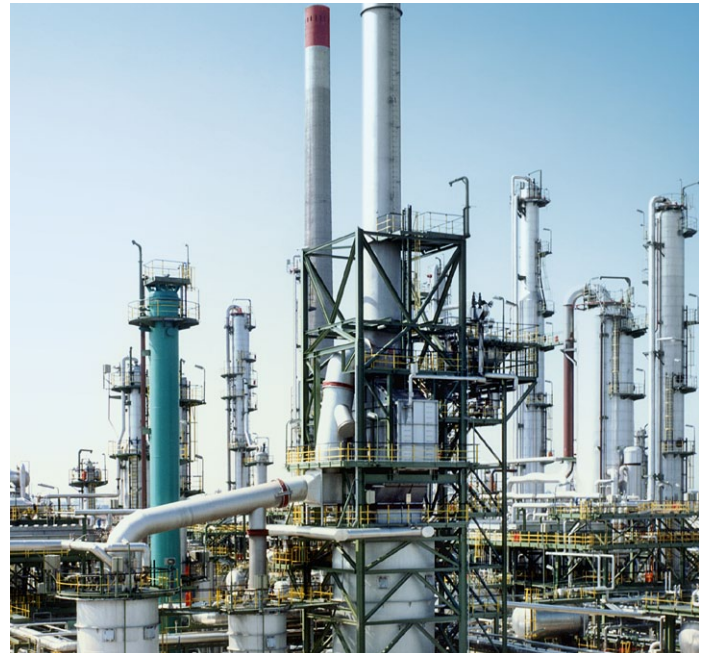
Figure 38: Furnaces for pre-heating products in a refinery
