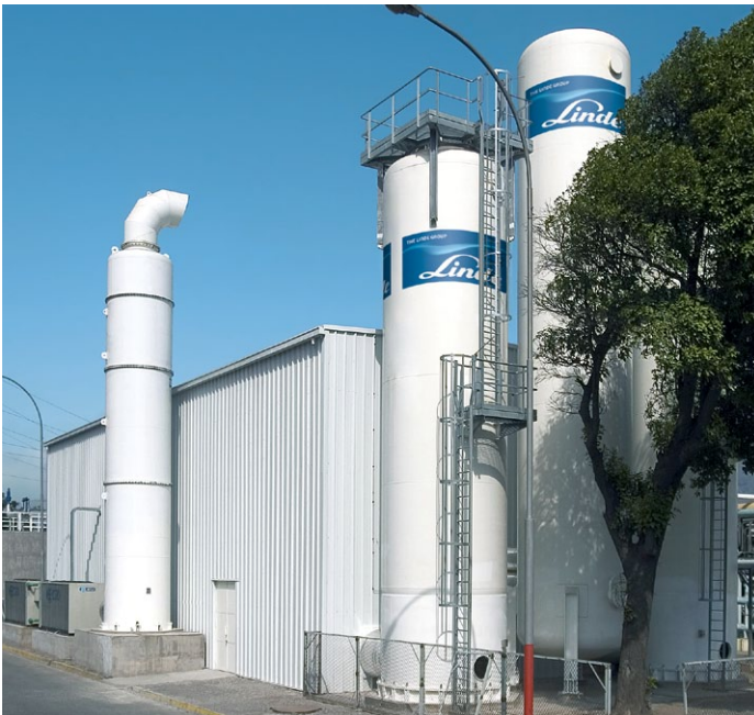
Figure 4: Adsorption oxygen plant
