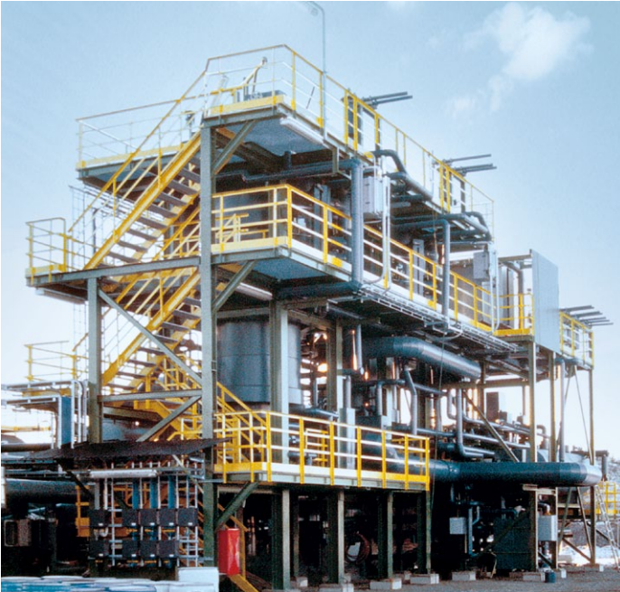
Figure 25: Claus plant with SURE burner
