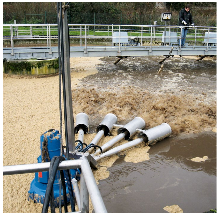
Figure 43: Venturi system for injecting oxygen into stabilisation ponds
