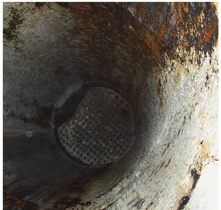
Figure 33: Corrosion caused by ammonia salt deposits
