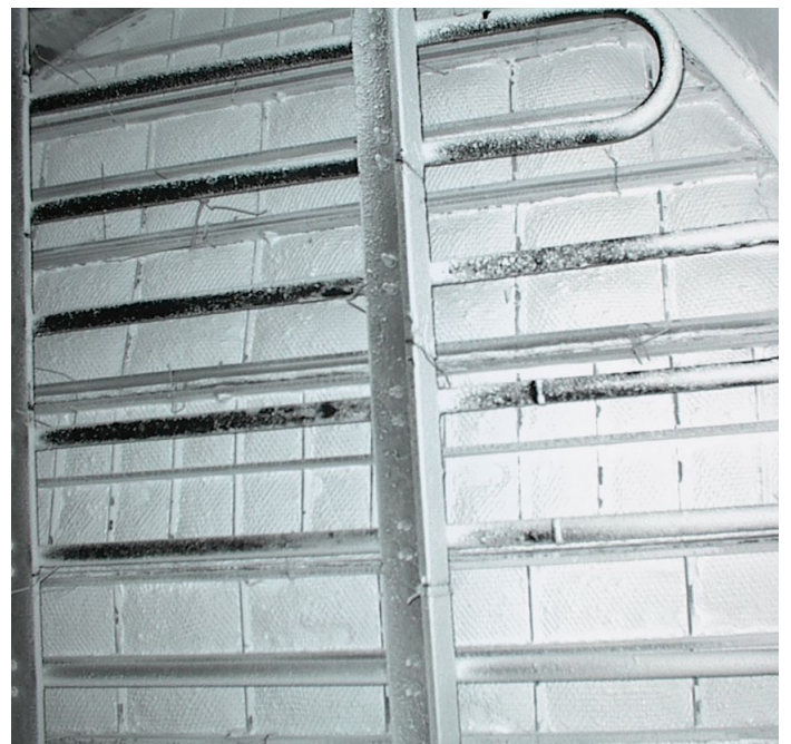
Figure 28: Demister with major ammonium salt deposits
