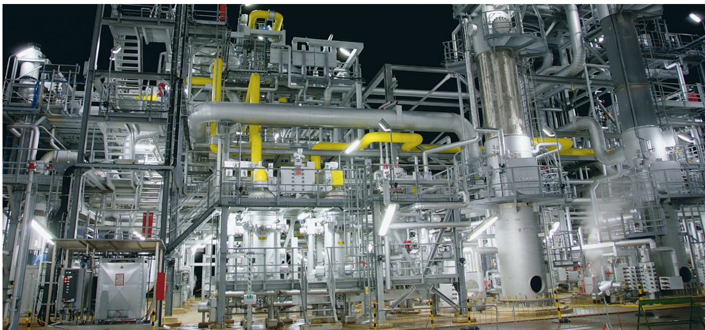
Figure 18: Modern Claus plant (With kind permission of Bayernoil Raffineriegesellschaft mbH. Photo taken by Jürgen Sturany.)
