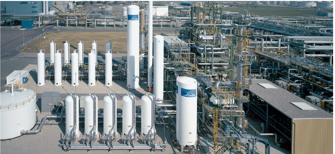
Figure 16: Crude oil refinery in Leuna with hydrogen plant
