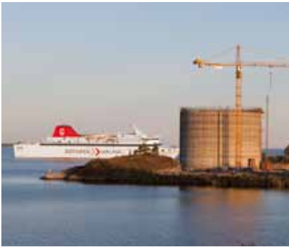
Full of energy: In Nynäshamn, liquefied natural gas is stored in special tanks built by Linde Group member AGA, from where it is transported to various customers.
