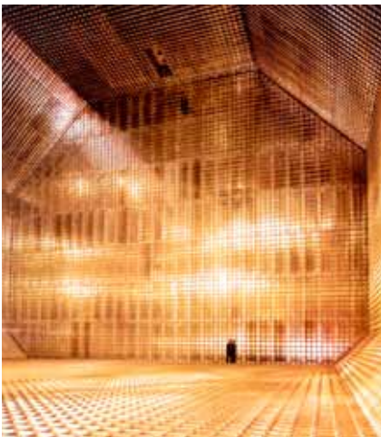
Insulated hold: Membrane tankers are built with high-grade steel and layers of insulating material for efficient, safe storage of LNG.
