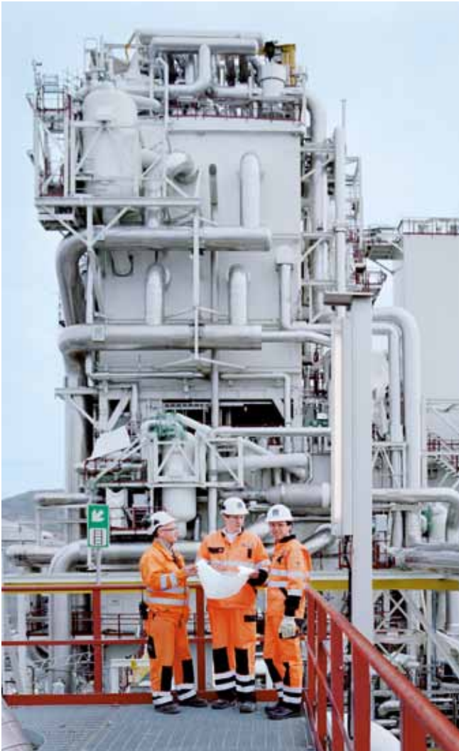
Giant jigsaw: The individual plant modules for Hammerfest were preassembled at different locations across Europe. These giant steel components were then transported thousands of kilometres on huge ships to the north of Norway. Linde engineers supervised local assembly, ensuring the gas turbines, pumps, compressors and heat exchangers dovetailed to perfection.
