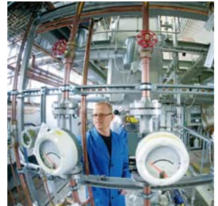
Overview of all processes: an employee of the Vattenfall pilot plant reviews the data from individual process steps.
