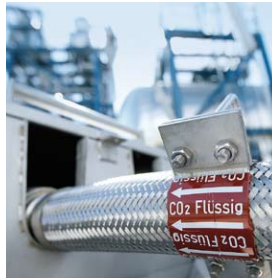
Securely transporting and storing: carbon dioxide from the flue gas that accrues in Schwarze Pumpe is taken by tank truck 400 kilometres to the Altmark and there injected into an exhausted natural gas field.
