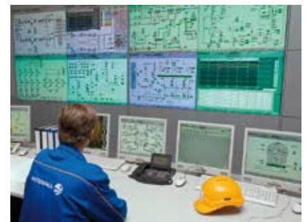
Pilot plant under control: with a modern process control system, the Oxyfuel process can be closely monitored.
