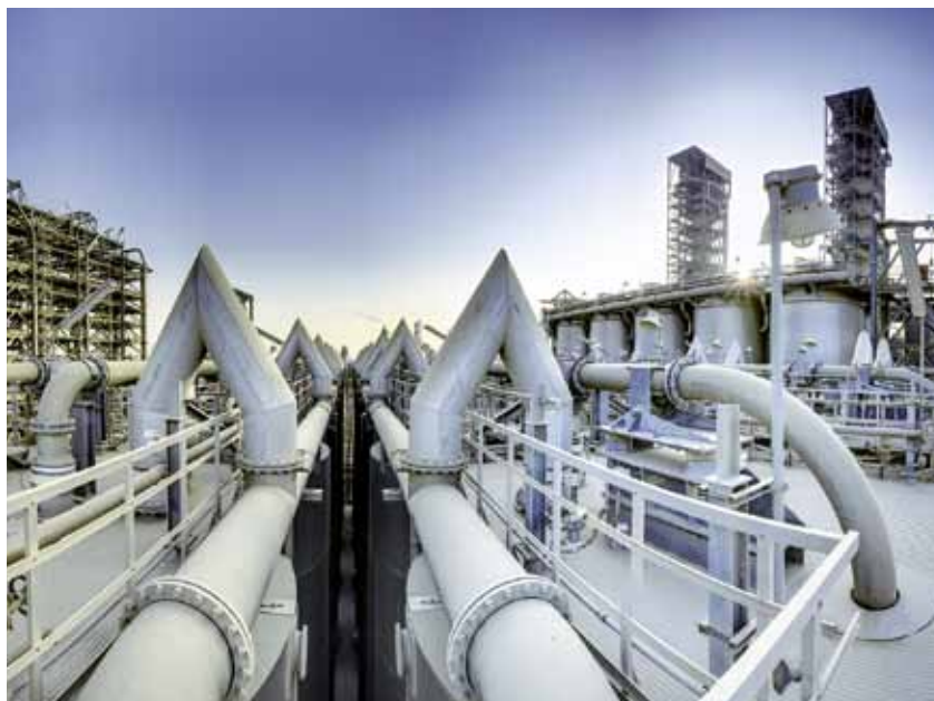
Polymer pipelines: Ethylene gas is converted into the widely used PE plastic at the polyethylene plant in Al Jubail, Saudi Arabia (right). This is then used to make plastic bottles (left) as well as a wide range of films, fibres, cables and moulded parts.
