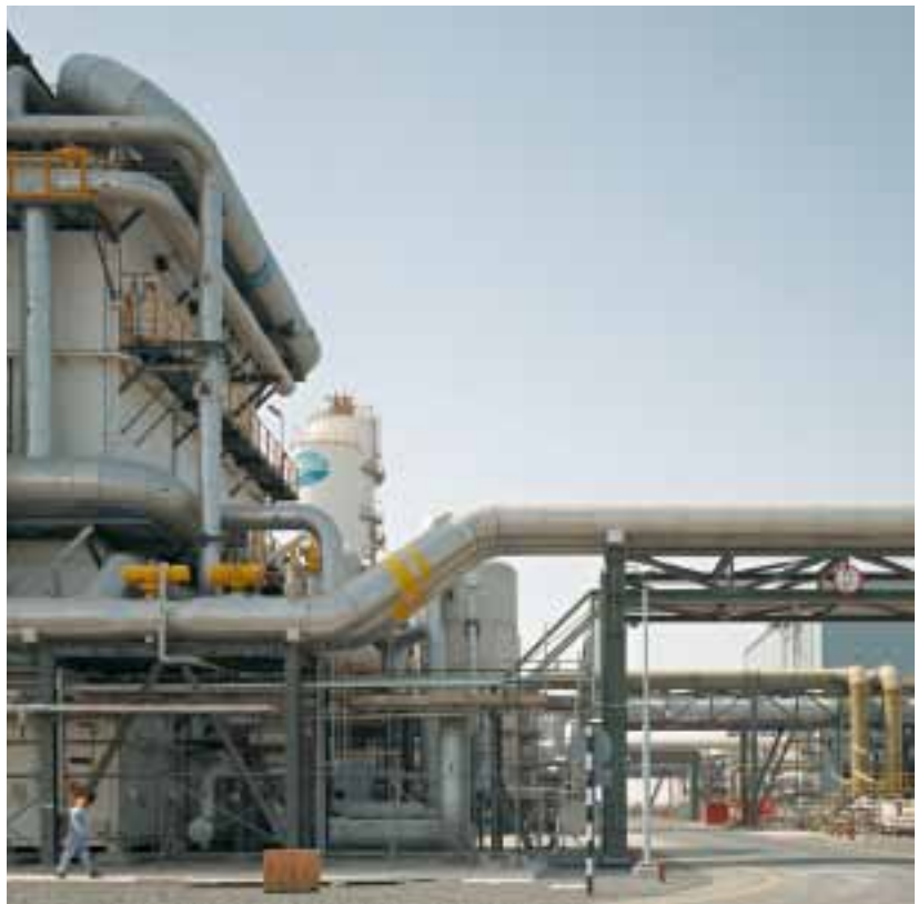
↳ Elixier II in action: The air separation plants at Mirfa, Abu Dhabi, were designed and built by Linde's Engineering Division.
